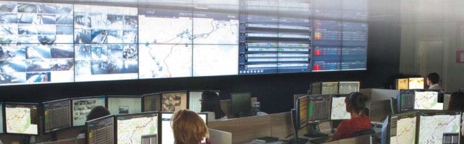
CCO - Belo Horizonte, MG, Brasil (3.100 ônibus e 42 companhias operadoras). Operational Control Center - Belo Horizonte, MG, Brazil (3,100 buses and 42 operator companies).
